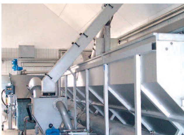
Intensive washing of screenings in a WAP® SL subsequent to a HUBER Complete Plant ROTAMAT® Ro5
